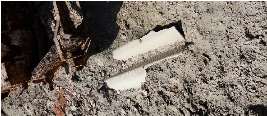
Photograph 6.4: Suspected Asbestos sheeting
