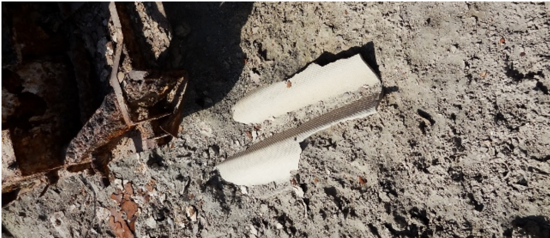
Photograph 6.4: Suspected Asbestos sheeting
