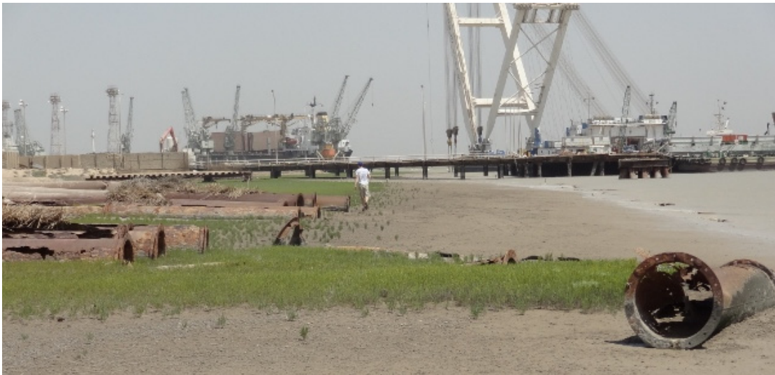
Photograph 6.2: Looking northwards along the intertidal zone towards KAZ Jetty No. 1. Please note the redundant pipework.
